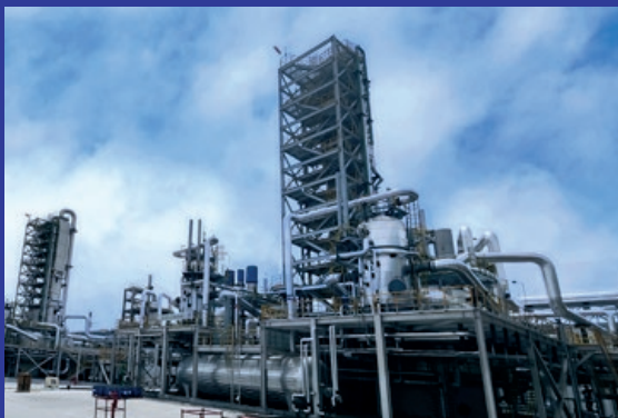
Three plants for Inner Mongolia Junzheng Chemical Industry Co., Ltd. in Inner Mongolia, China were all started up in one go in June of 2024.
