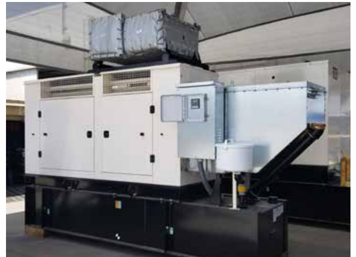
ActivDPF on 400 kW genset using 200 kW radiator-cooled load bank
