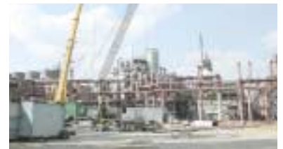
The new Perstorp Formox plant was in the final stages of construction at the time of this photo in September.
