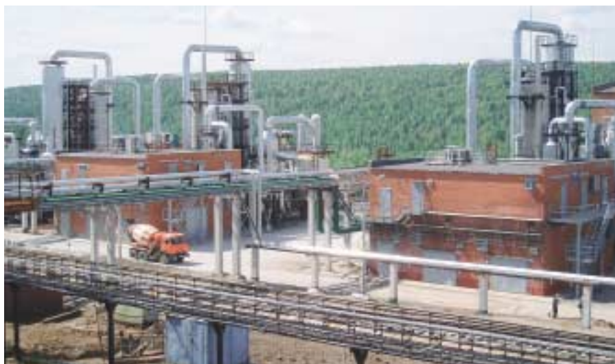
Three Perstorp Formox plants at the Metafrax site in Gubakha, where winter temperatures can reach -50^{\circ}\text{C}
