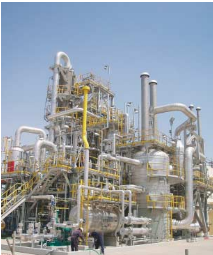
SAFCO's new UFC plant
