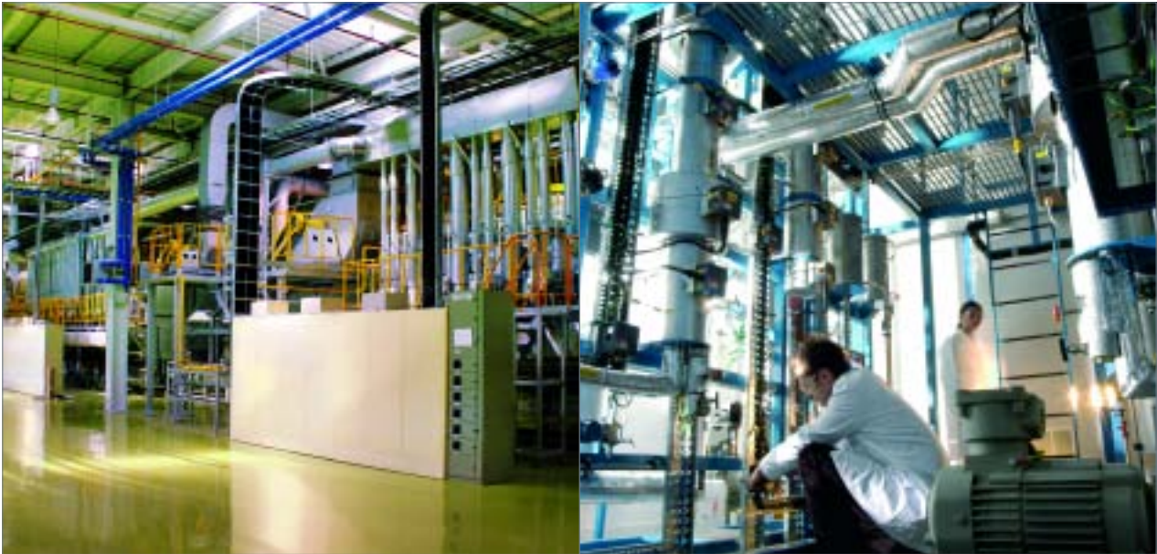
Above: Johnson Matthey's new catalyst manufacturing plant in South Korea will begin production during 2007/08.
