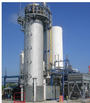
Figure 1. Air Liquide steam methane reformer unit in Roussillon, France
