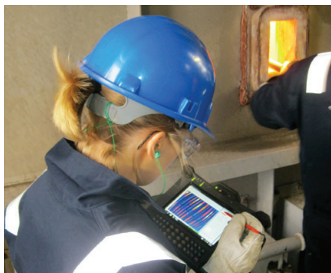
Above: Live thermal footage of the reformer internal is reviewed by our reformer engineer to ensure good quality data is collected on-site.
