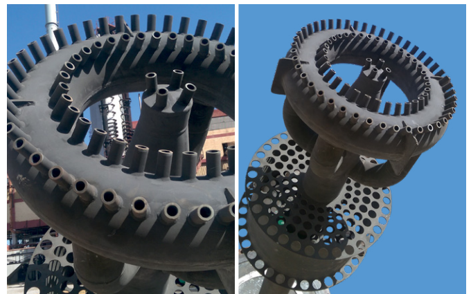
Burner after 6yrs of operating with no damage
